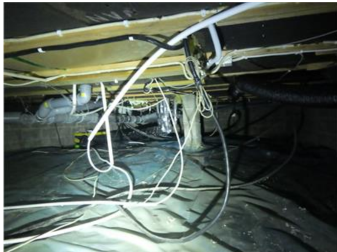
Elinstallationer i kryppgrund.
